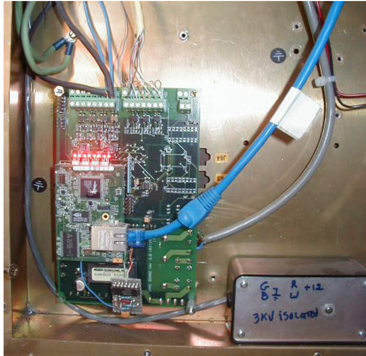
Figure 34: Interface board connected to lights
